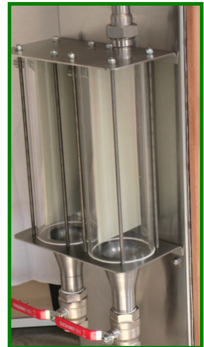
Two-stage sedimentation unit
